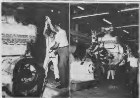
WHEN LAGO began using governmental power, six of ten steam turbo-generators in Powerhouse No. 1 were declared surplus and dismantled. Among those were the three installed when the powerhouse was erected in 1922 during Lago's early development.
